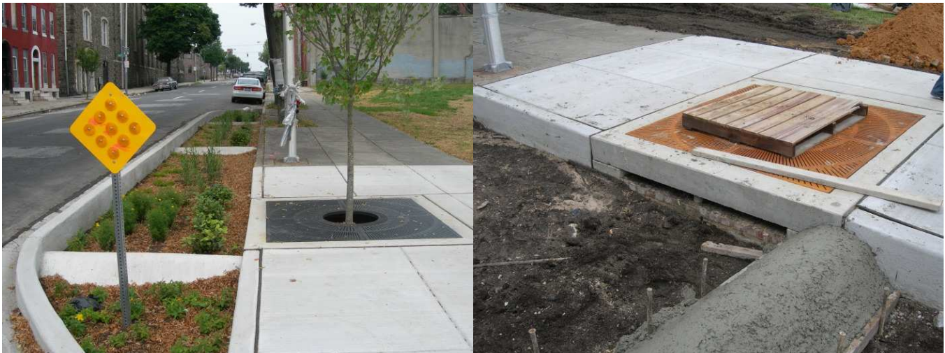
DPW Curb Extension in sub-drainage area "O", Baltimore Street, in Franklin Square neighborhood. Printed with permission from the Parks & People Foundation.
