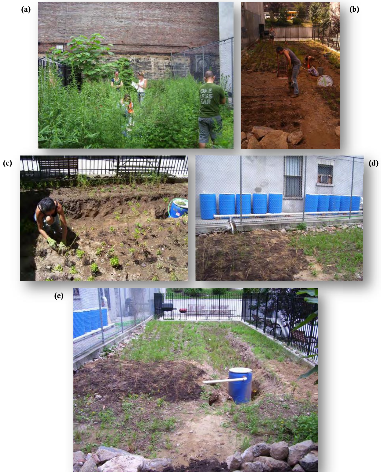
Figure 10. 150 th Street Project. Site before project (a), site prep (jackhammering the soil) (b), planting (c), rain barrel hookup (d), rain garden and rain barrel float switch installation (e). Photo credit: Tatiana Morin with New York City Soil Water Conservation District.
